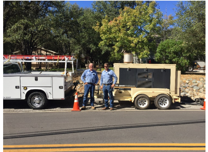
NID electrical systems technicians set up a generator in advance of a power shutoff in October.
