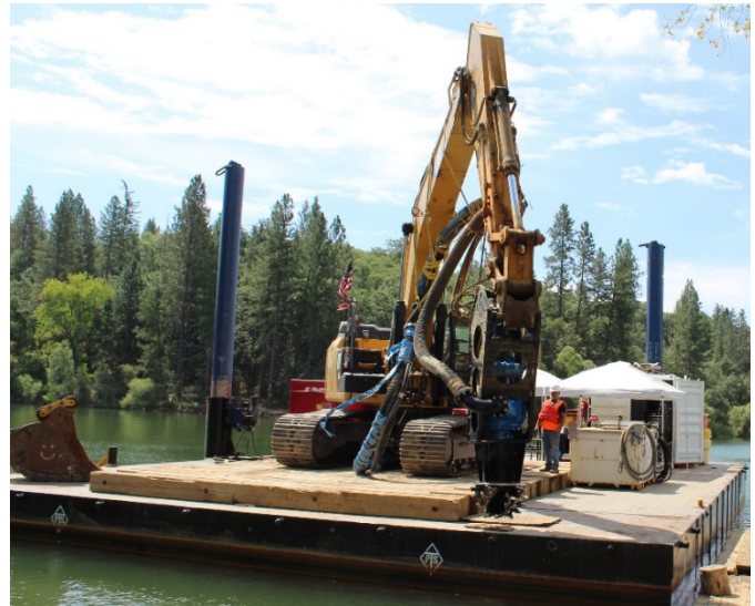
From Combie Reservoir a suction dredge removed wet sediment for the centrifuge process.
