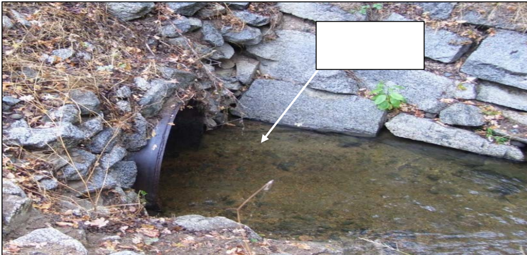
PHOTO 3-3 CANAL CULVERT OUTLET WITH ACCUMULATED SEDIMENT
