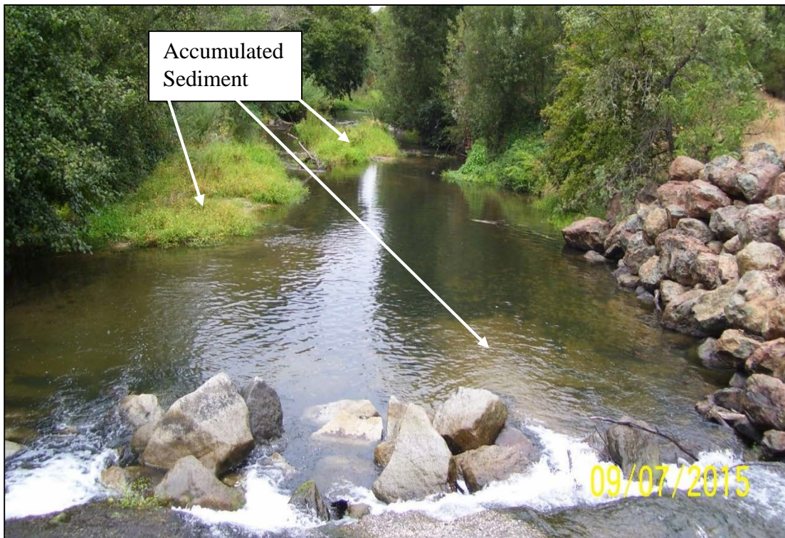
PHOTO 3-8 DOWNSTREAM VIEW OF DIVERSION STRUCTURE WITH SCOUR POOL, SEDIMENT ACCUMULATION, AND DEBRIS
