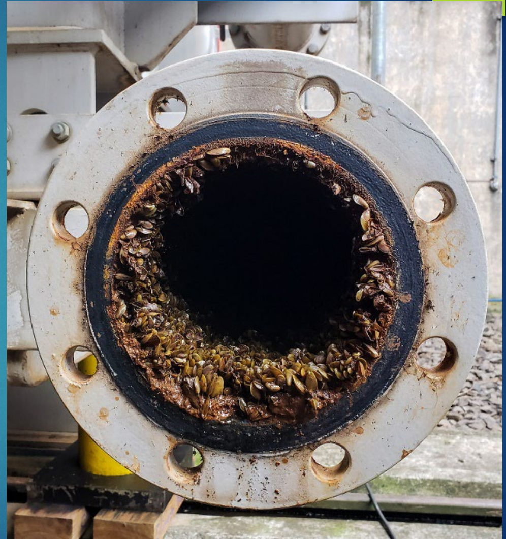
Figure 2: Golden Mussels colonizing a water pipe at a hydroelectric plant in Brazil (Mountinho, 2021).
