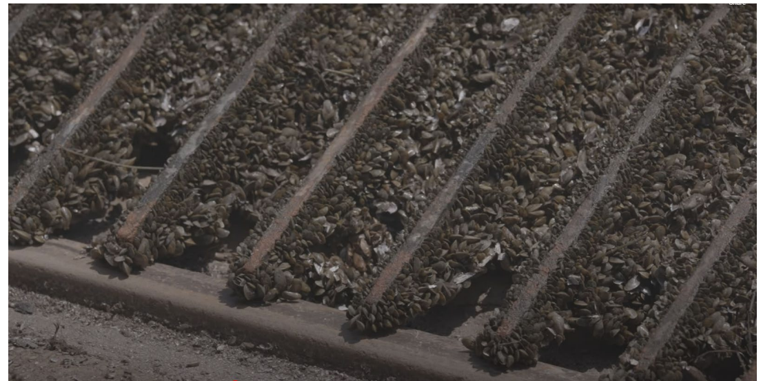
Figure 18: A colony of golden mussels ( Limnoperna fortunei ) on a hydroelectric powerhouse intake rack, Brazil.
