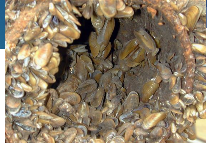
Figure 13: Golden Mussels fouling on an iron pipe.
