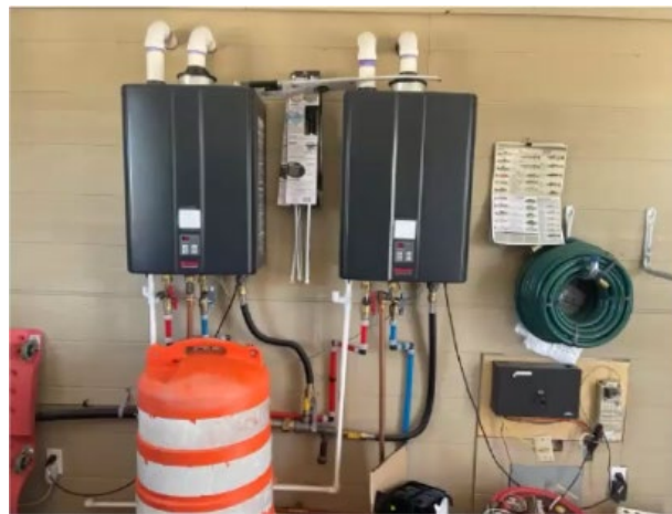
Figure23: On-Demand hot water decontamination unit
