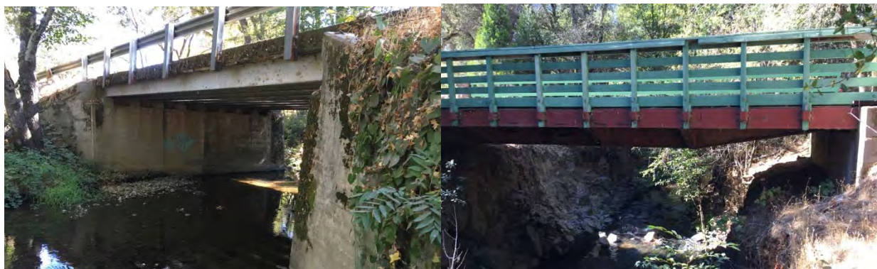
Figure 4-7: Bridge Crossing on Rough and Ready Highway (Left), and Bridge Crossing on Cook Road (Right)
